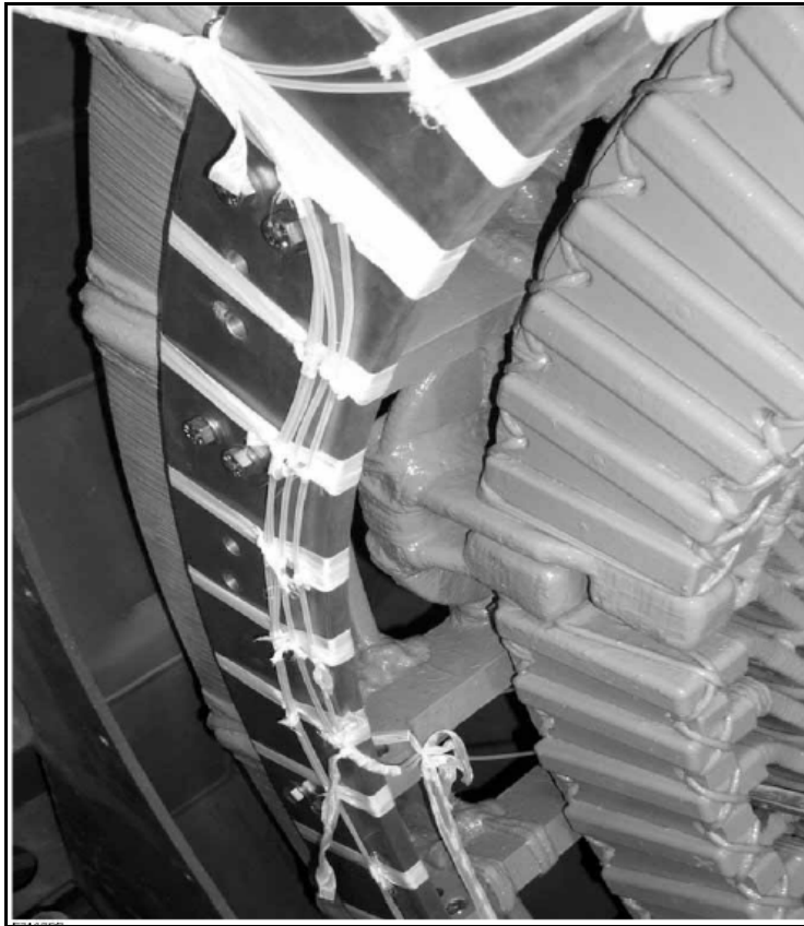
Other example of fiberglass ties and bundling of fiber optic cables FIGURE 6
