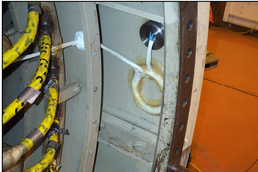
Managing excess cable in hydrogen-cooled turbo-generators FIGURE 7
