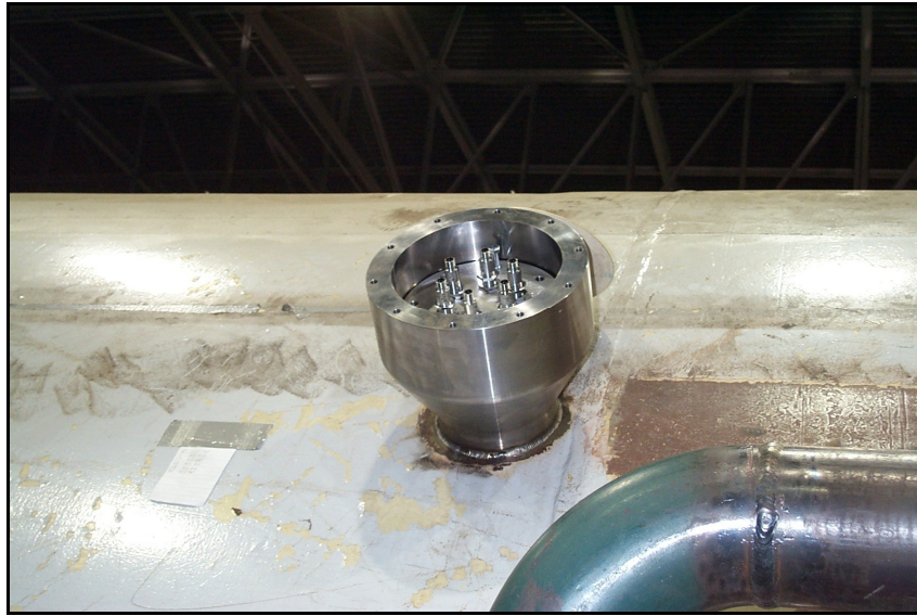
Sealed flange with six conditioners installed FIGURE 8
