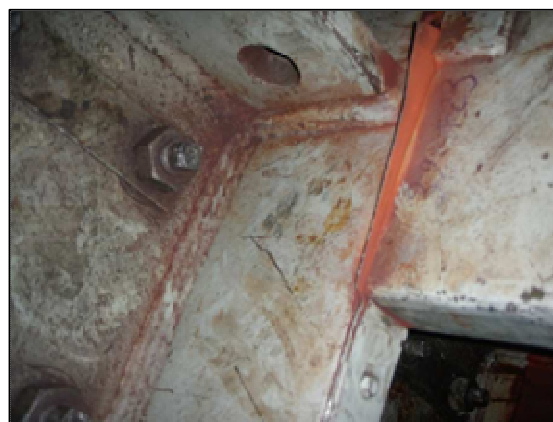
Fretting corrosion at rim/hub junction.
